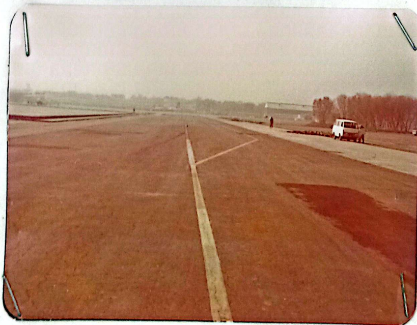
4 VIEW OF APRON FROM TAXIWAY NO.1. THE PASSENGER PALLET WAS LYING FEW FEET RIGHT OF THE VEHICLE.
