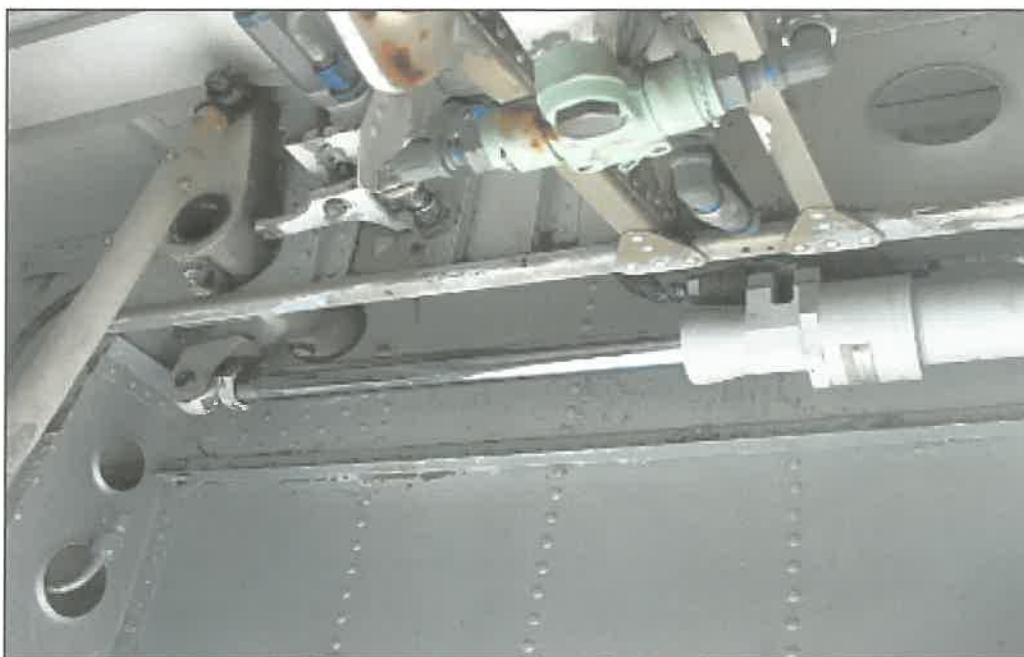
APPENDIX K10 NOSE LANDING GEAR ACTUATOR IN FULLY EXTENDED POSITION – NO EVIDENCE OF HYDRAULIC LEAK
