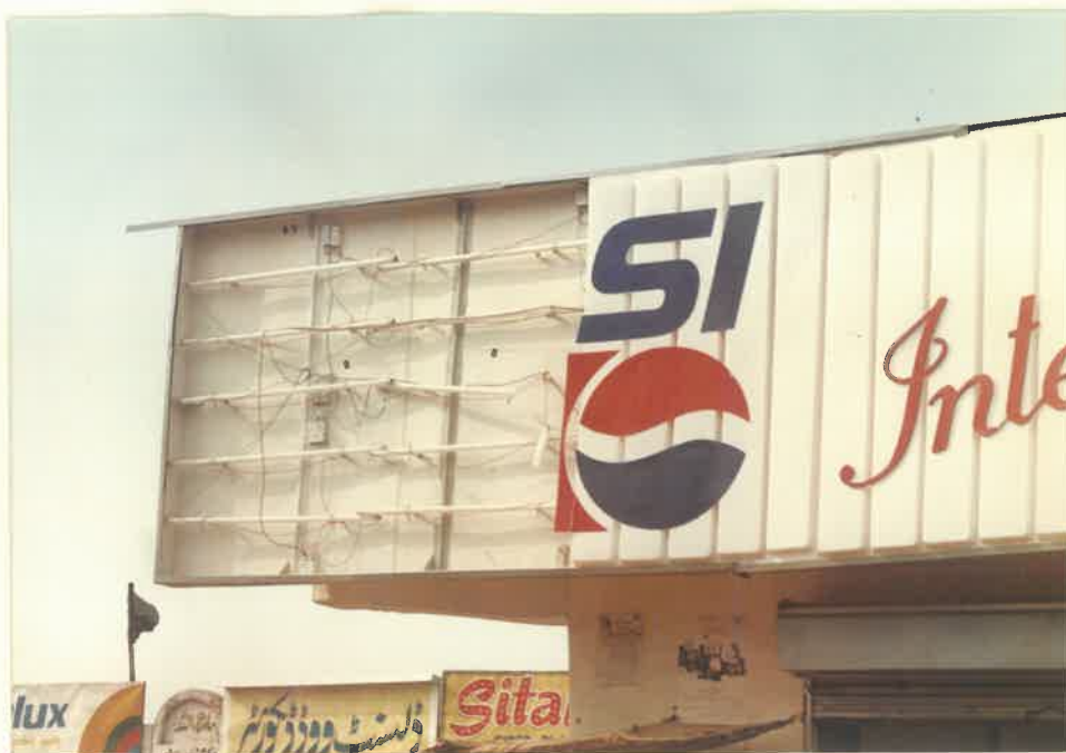
11. DAMAGES ACROSS JAMRUD ROAD SIGN BOARD
