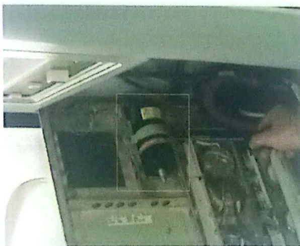
Oxygen chemical generators. The orange strip turns black when the generator is once used.
