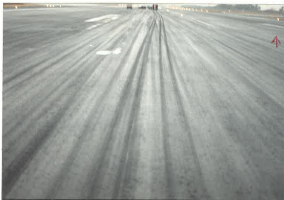
TYRE MARKS BETWEEN 500 - 1000 FEET BEFORE THE STOPPING POINT OF A/C
