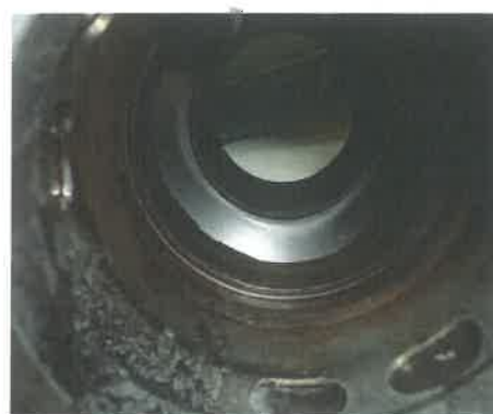
Internal view of No.2 bearing housing
