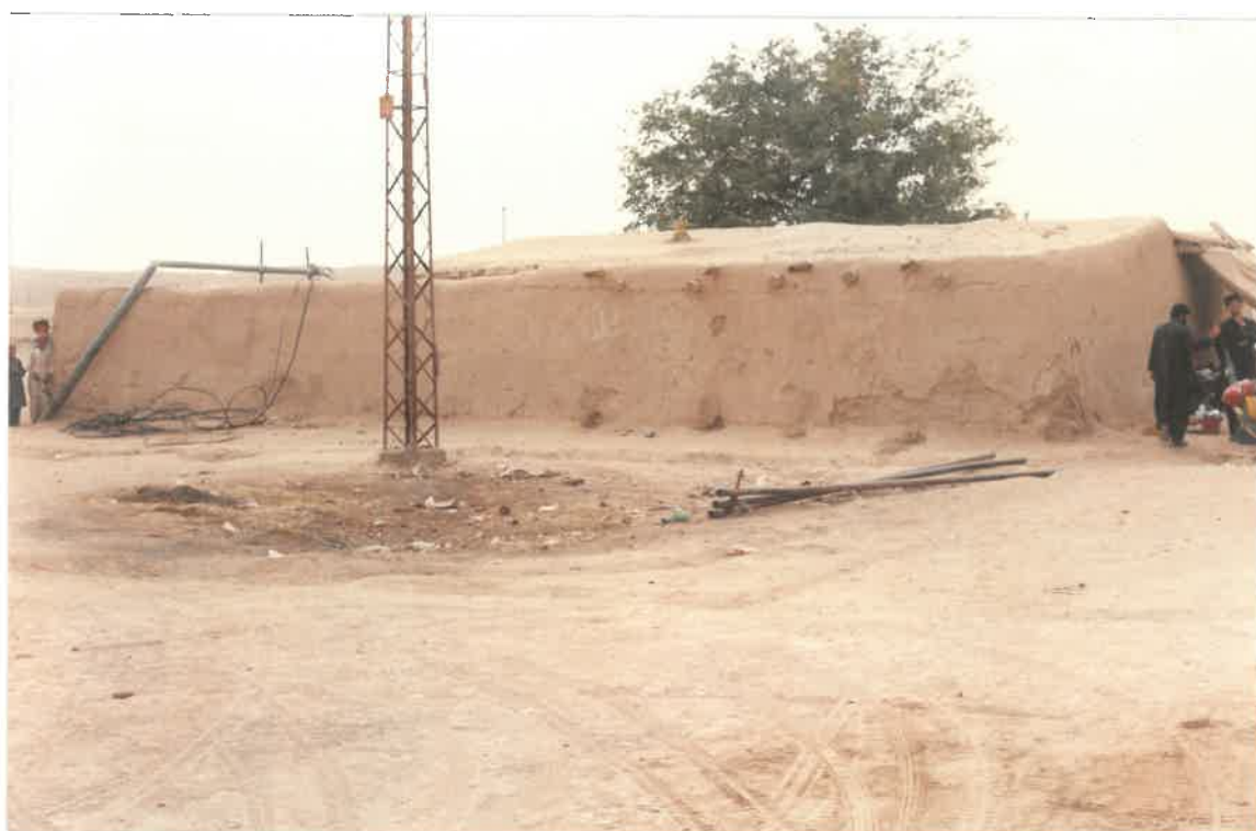
BENT TELEPHONE POLE ON LEFT EDGE INDICATIVE OF 'PULL' FORCE ON THE TELEPHONE MULTI-CABLE
