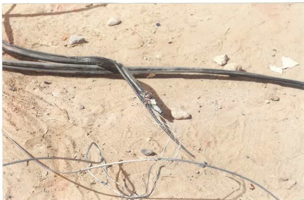
BROKEN TELEPHONE MULTICABLES
