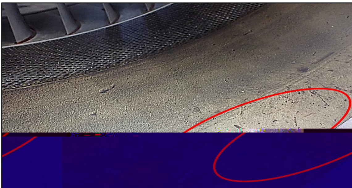
Figure 3 Scratch marks on Fan Case Assembly
