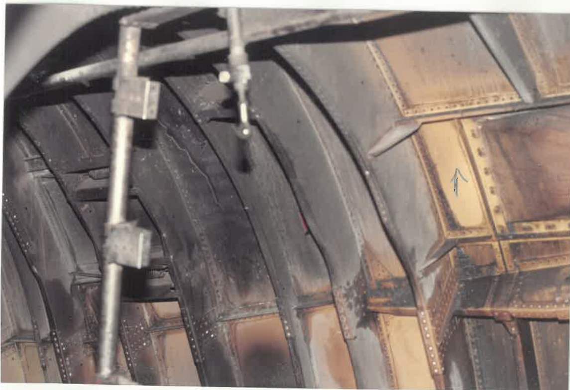
FIRE DAMAGE EVIDENCE INSIDE VIEW
