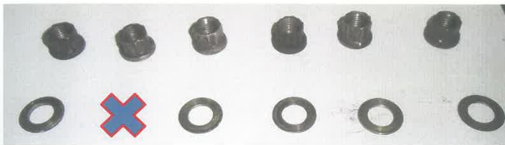
One Washer Found Missing
