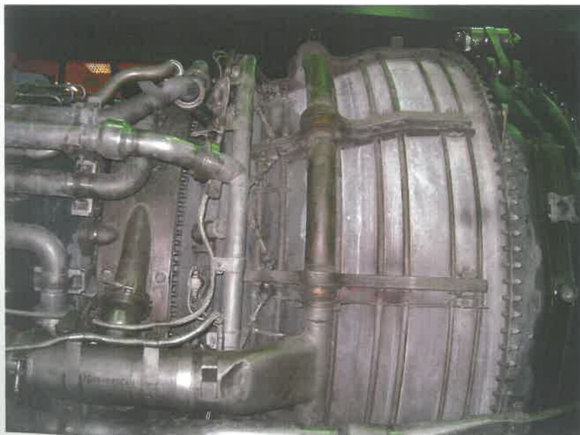
High Pressure Turbine and Low Pressure Turbine Casing
