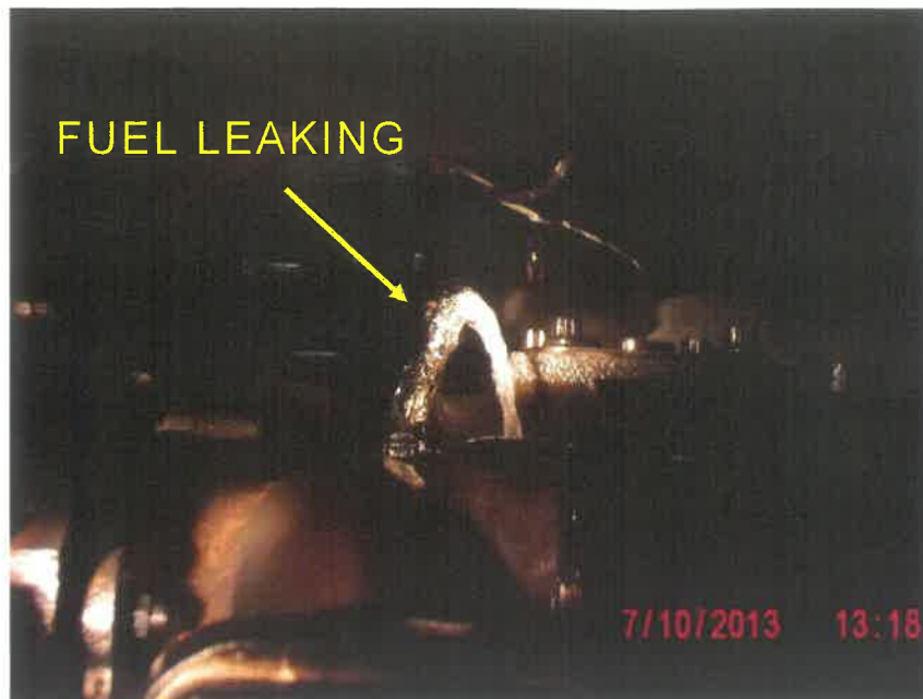
Fuel Leaking from Top of MEC Under Gravity
