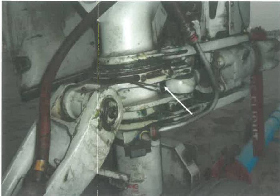
The lower end of broken steering cable on steering collar
