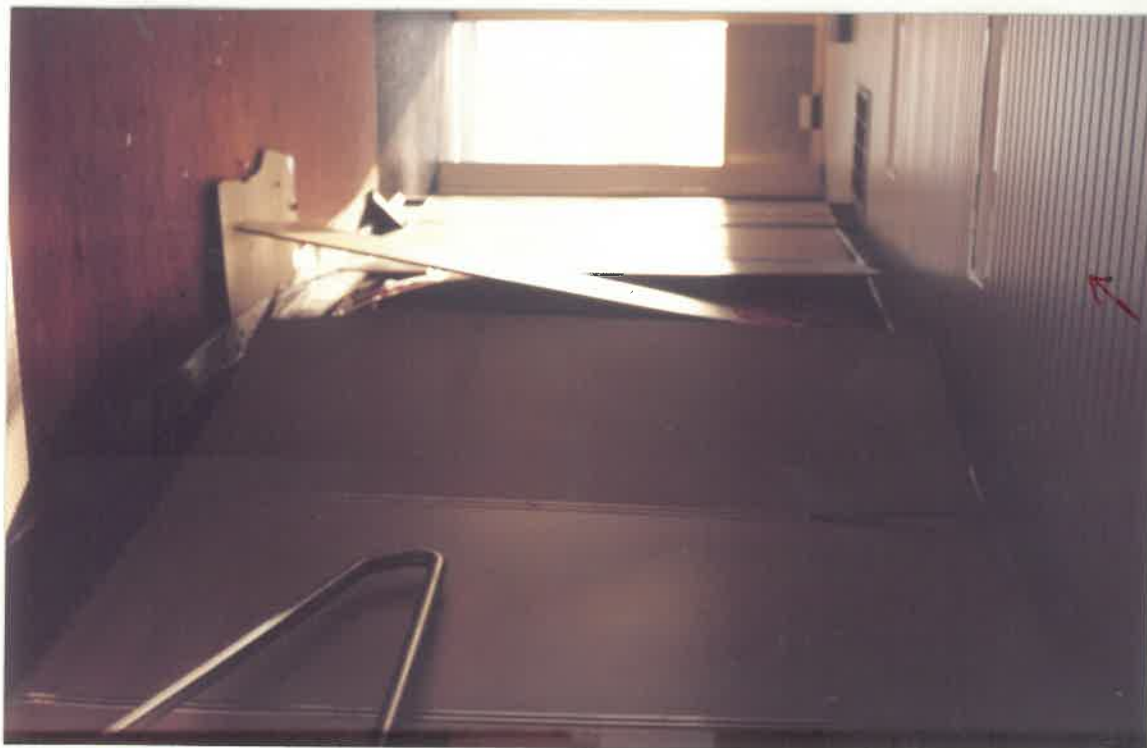
AVIOBRIDGE NO. 25 INTERNAL DAMAGE TO SIDE WALL AFTER THE INCIDENT
