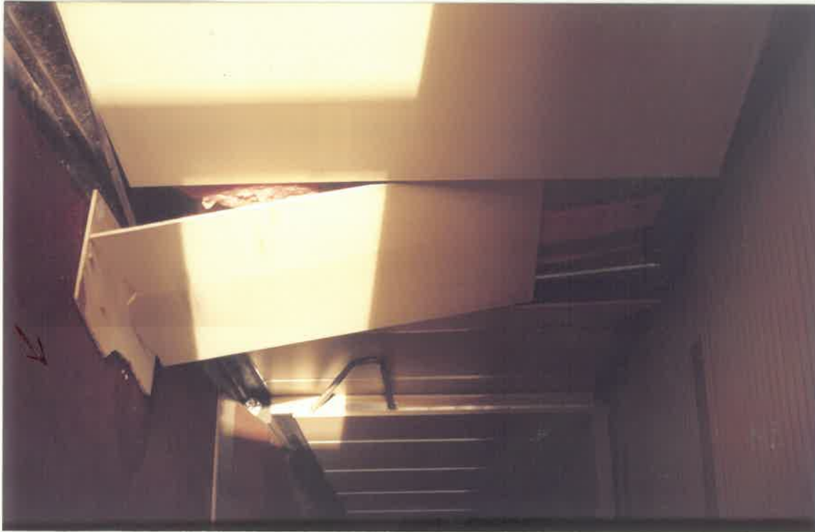
AVIOBRIDGE NO.25 INSIDE DAMAGE AFTER THE INCIDENT (ANOTHER VIEW)
