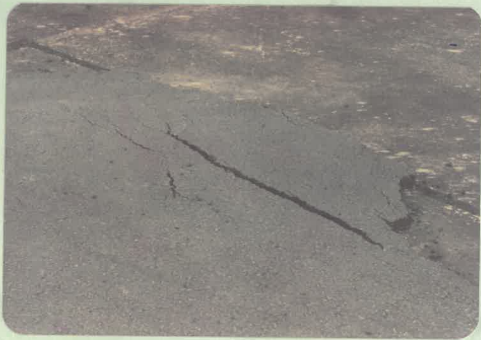
ANOTHER VIEW OF THE FAILED OVERLAY
